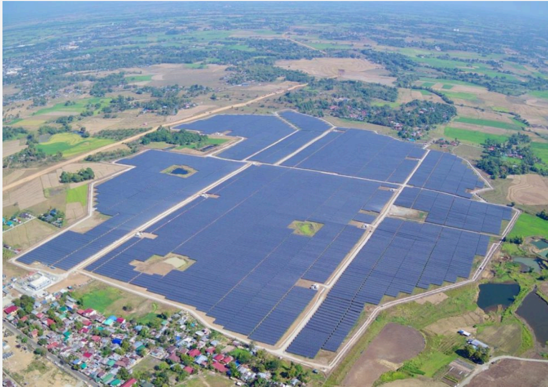
SOLAR POWER. The 50-megawatt BulacanSol solar power plant of PowerSource First Bulacan Solar, Inc. in San Miguel, Bulacan. BulacanSol starts providing additional renewable power to the Luzon grid. (Photo courtesy of MGen)
